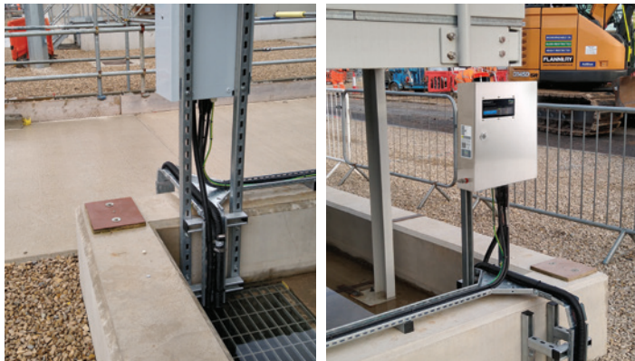
Special-build that interfaces with existing glycol alarm system.
